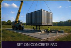
SET ON CONCRETE PAD
